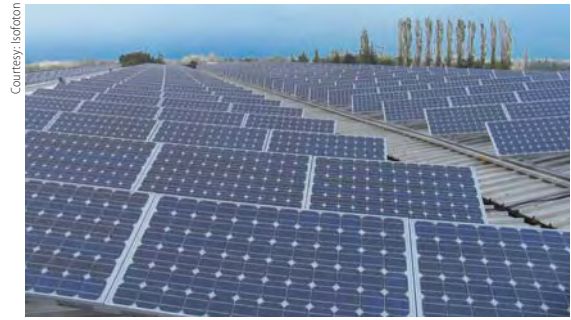
A solar PV roof top installation by Isofoton has cut costs at the Torelli Pierluigi cheese factory in Parma, Italy.
