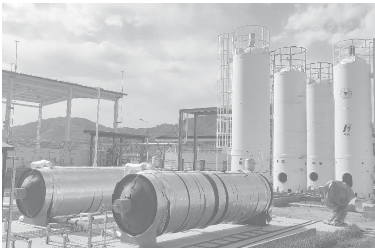
The 45 MPa high-pressure hydrogen storage facilities of Zhangjiakou Wangshan Hydrogen Production and Hydrogenation Station (photo: Hui Zhao, Hypower Hydrogen Technology Co., Ltd, 2020).
