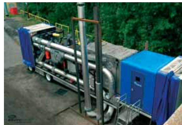
The EnviroScrub Technologies Mobile Unit running at the Potlatch Paper Corporation facility.
