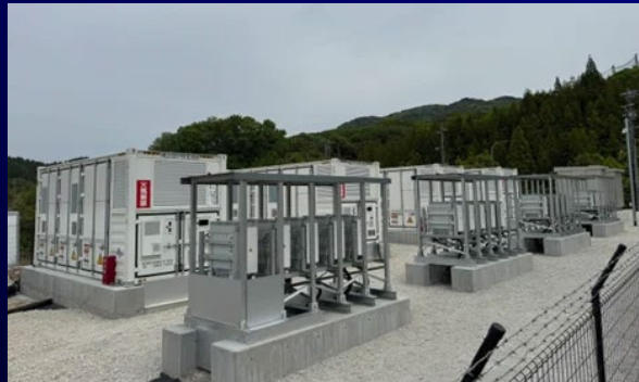
Stationery Battery Smart Grid Data Center
