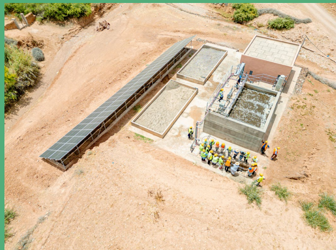
Construction of an HMB System in the Rural District of Al Haouz, Morocco
